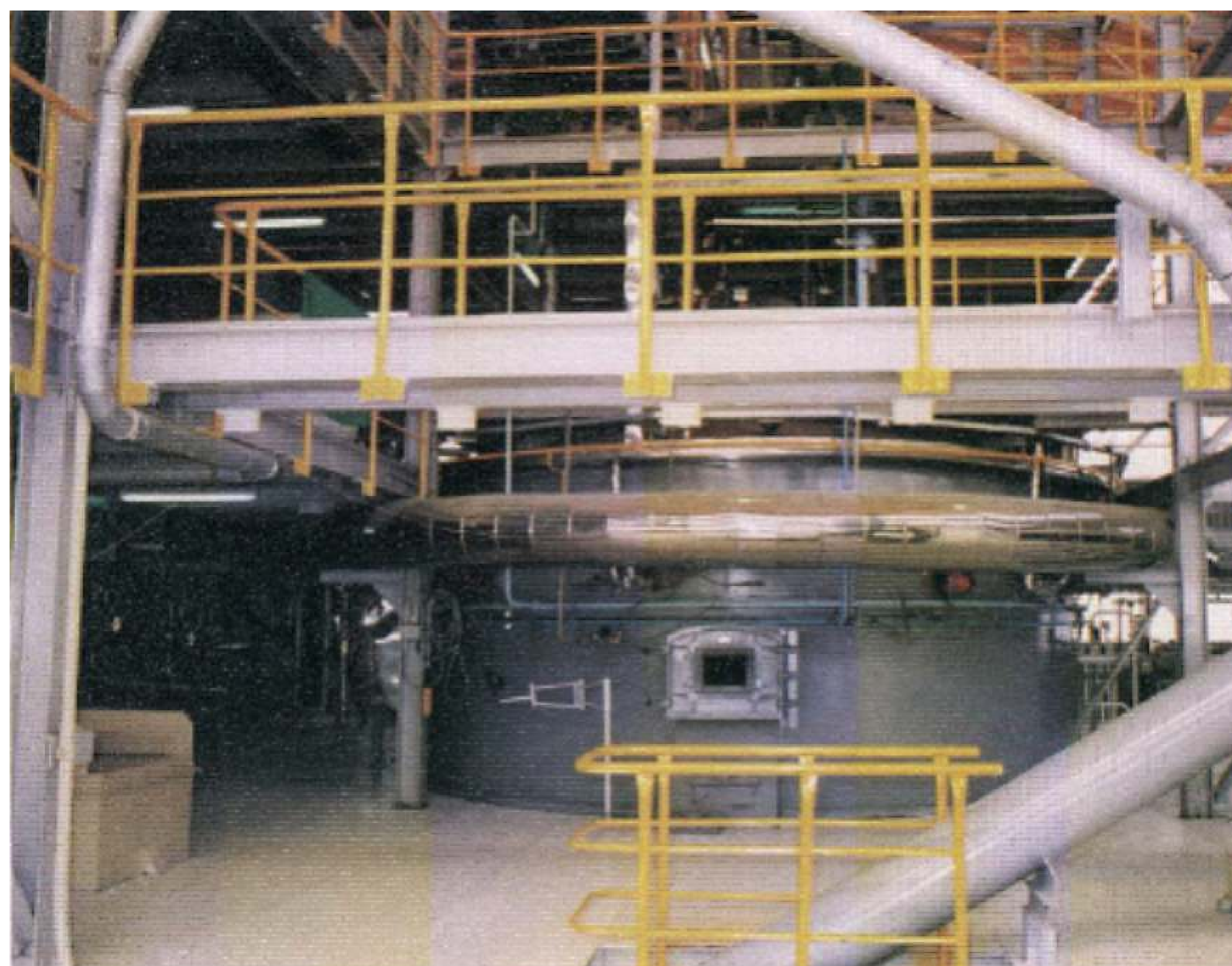
Total view of furnace system
